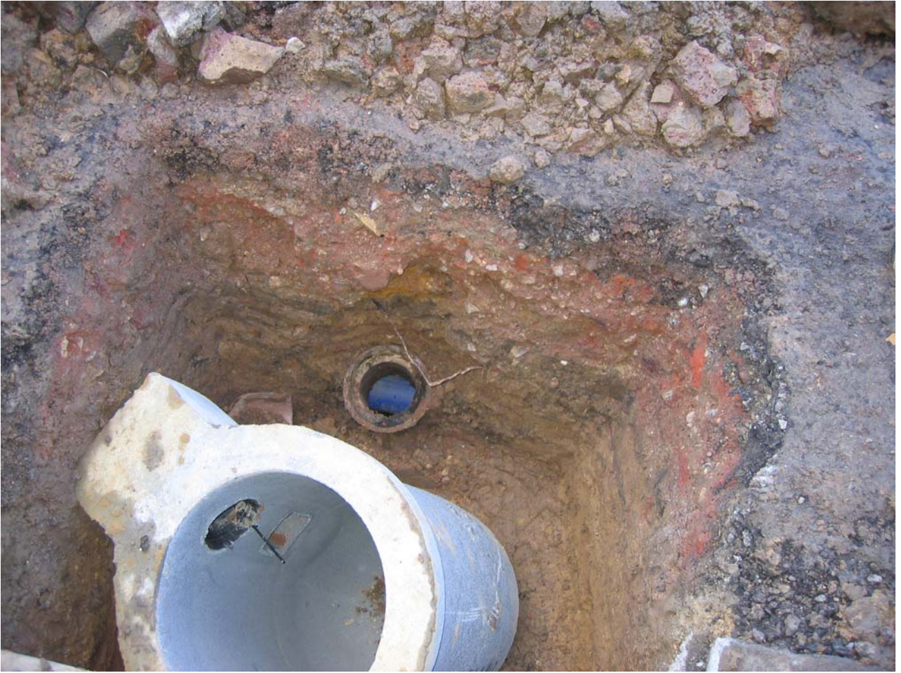
Severed gully connection.
